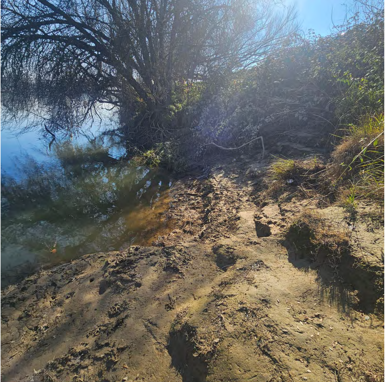
Erosion site along the Sacramento River across from the condominium complex Riva's of the River (February 2026)
