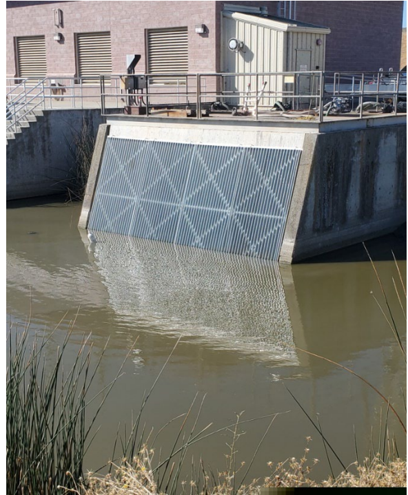
New trash racks
