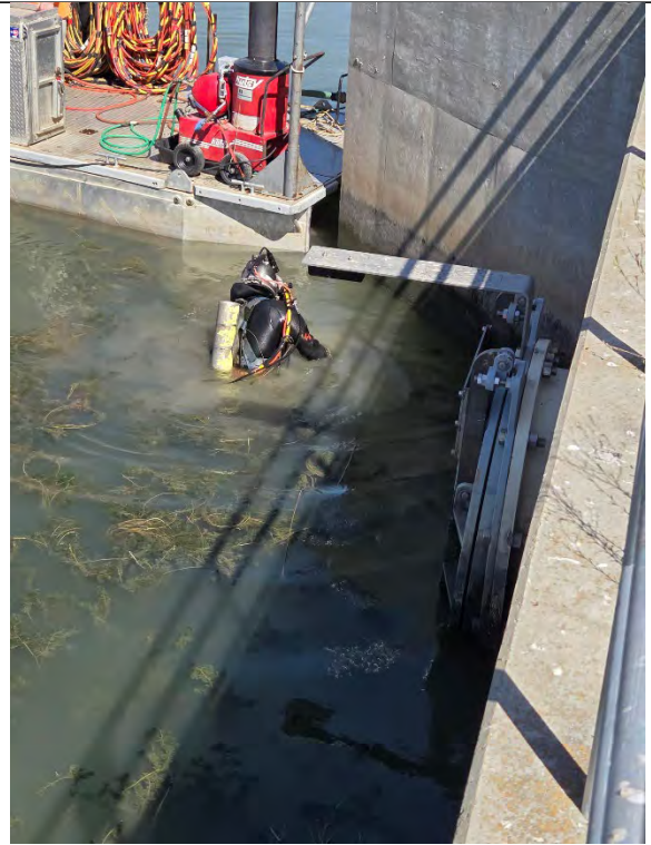
Diver in water at pump station discharge pipes
