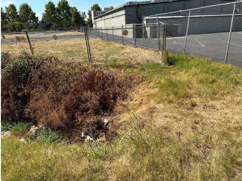
Ditch behind Bowling Alley
