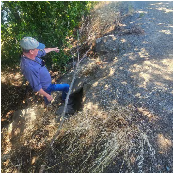
Hole found on Sacramento River levee (has been repaired)
